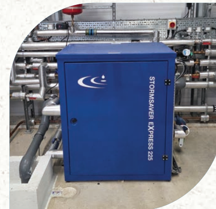
Rainwater harvesting system
