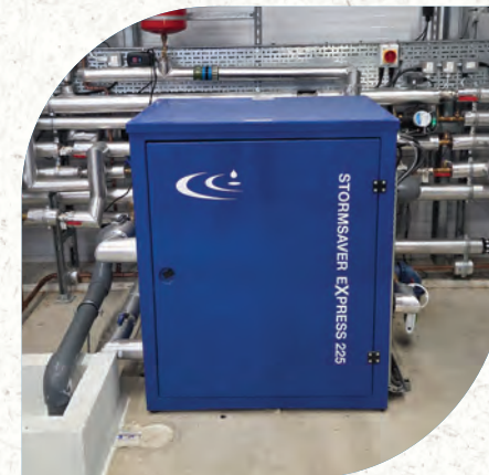
Rainwater harvesting system
